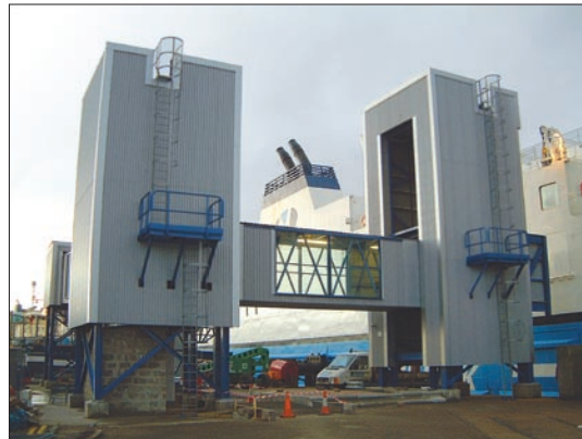
(Above) Isleburn Mackay & Macleod completed the preferred design for the Aberdeen Ferry Bridge by using Nook 50-ton ball screw jacks with 26-foot lifting shafts.
